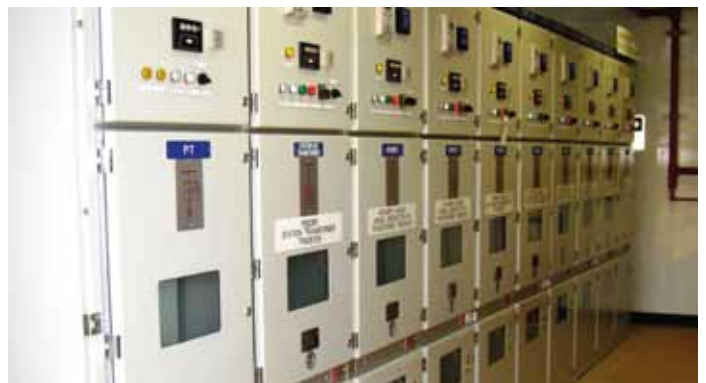
Switchgear (Switch room)
