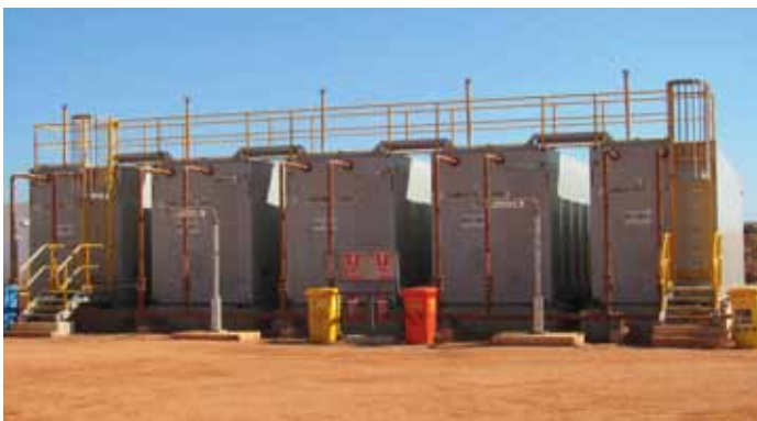
Fuel tanks & Fuelling systems
